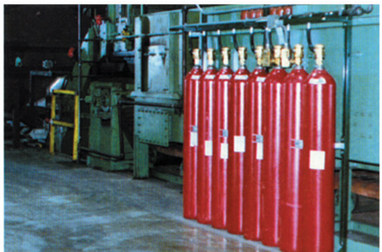
Local application protection for an industrial quench tank operation.
